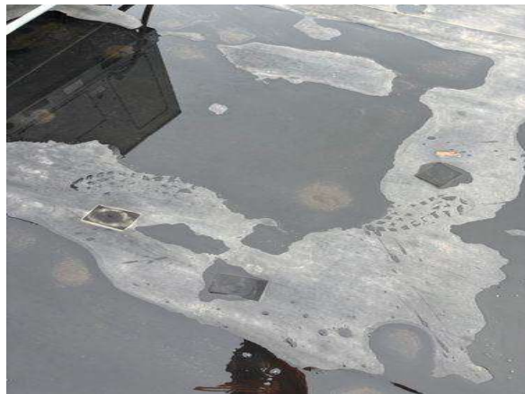
This is not the proper repair to patch an EPDM roof membrane.
