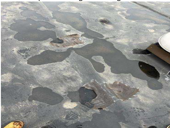
This is not the proper repair to patch an EPDM roof membrane.
