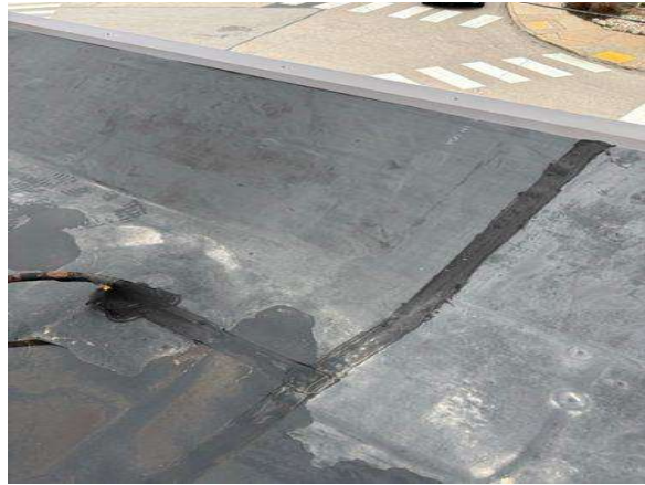
Whoever made these repairs cut 6" cover tape in half to seal a seam. The minimum tape size for an EPDM roof is 6", it should not be any thinner to ensure the seam is sealed correctly.
