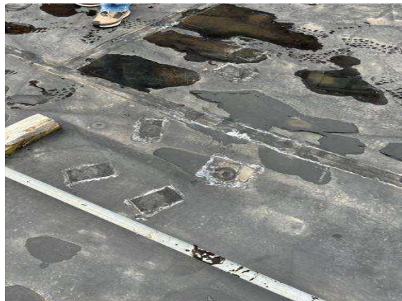
This is not the proper repair to patch an EPDM roof membrane.
