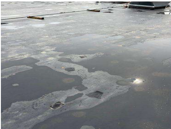
This is not the proper repair to patch an EPDM roof membrane.
