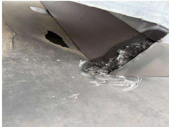
This is not the proper repair for metal flashing. Spray foam was used and then painted with what appears to be flex seal.
