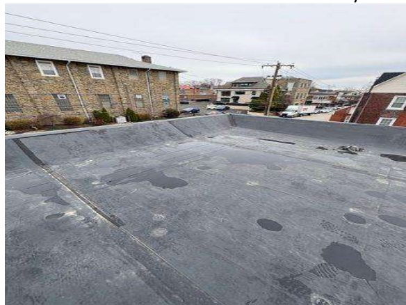
Whoever made these repairs cut 6" cover tape in half to seal a seam. The minimum tape size for an EPDM roof is 6", it should not be any thinner to ensure the seam is sealed correctly.
