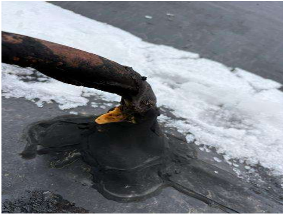
This conduit flashing is open and the spray insulation is exposed allowing water in.
