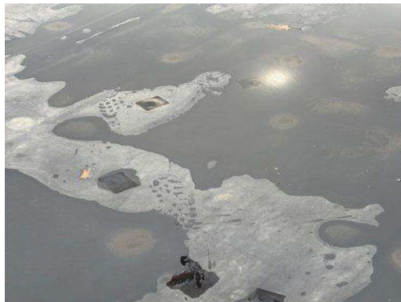
This is not the proper repair to patch an EPDM roof membrane.
