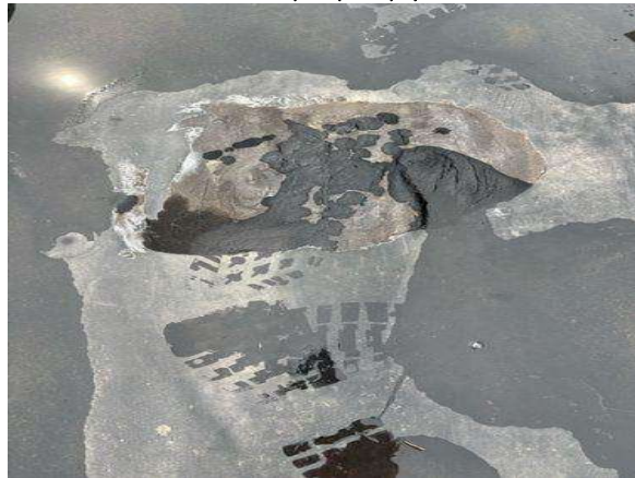
Roofing cement is not the proper repair material for an EPDM roof as the cement will eat away at the membrane over time.
