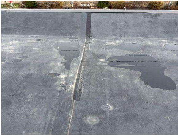
Whoever made these repairs cut 6" cover tape in half to seal a seam. The minimum tape size for an EPDM roof is 6", it should not be any thinner to ensure the seam is sealed correctly.
