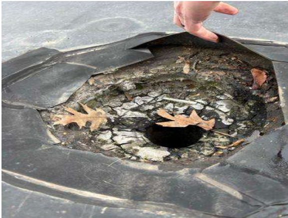
The roof material in the drainage areas are wide open allowing water to get in.
