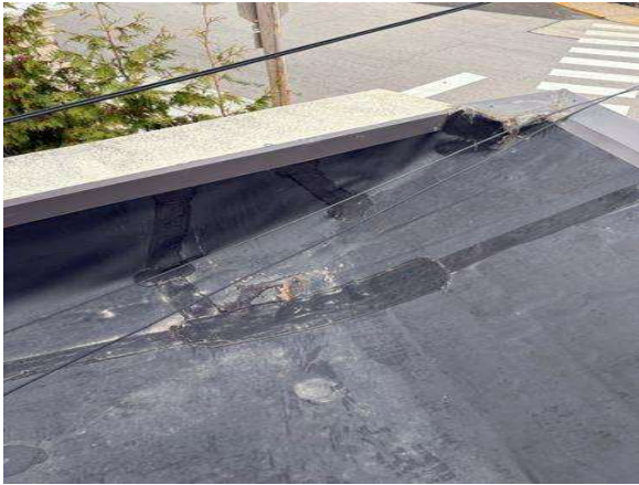
Whoever made these repairs cut 6" cover tape in half to seal a seam. The minimum tape size for an EPDM roof is 6", it should not be any thinner to ensure the seam is sealed correctly.
