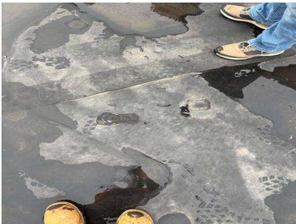
This is not the proper repair to patch an EPDM roof membrane.
