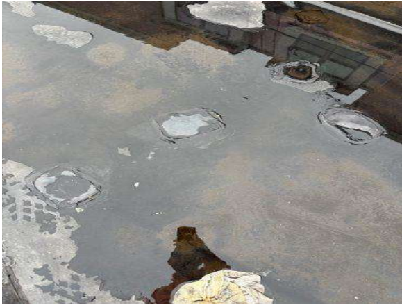
This is not the proper repair to patch an EPDM roof membrane.
