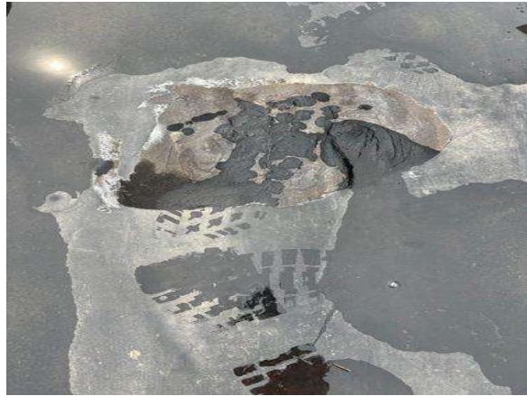
Roofing cement is not the proper repair material for an EPDM roof as the cement will eat away at the membrane over time.
