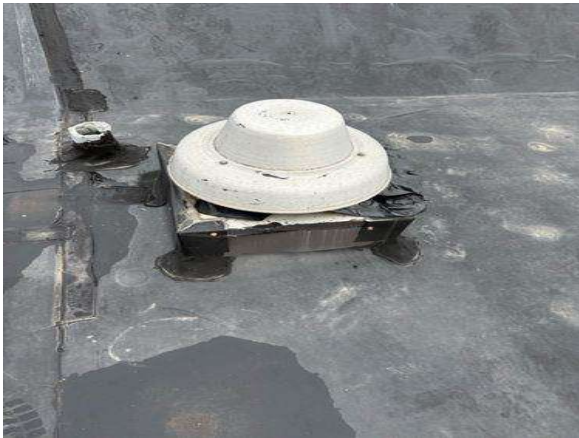
The corners of the metal are open.
