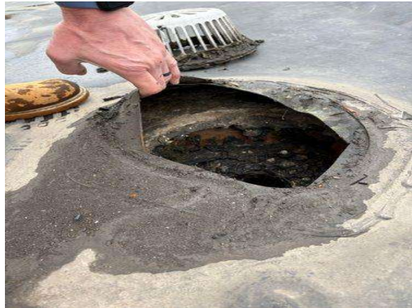
The roof material in the drainage areas are wide open allowing water to get in.
