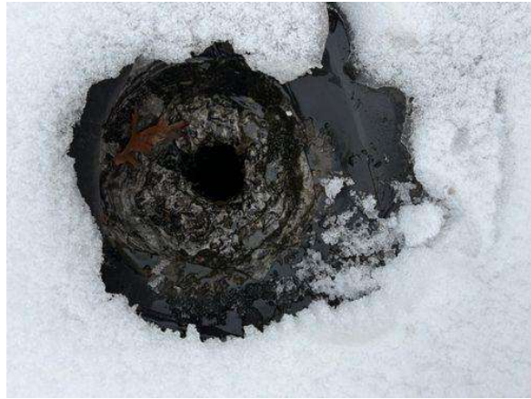
The material on this drain should be sealed with an O ring that the drain cover mounts on to keep the water out. The drains on this roof do not have that. See attached detail.
