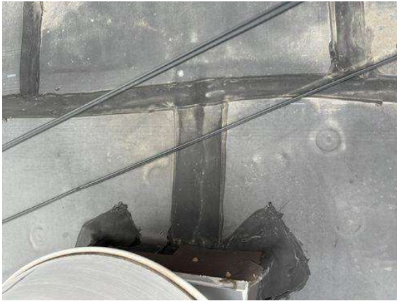
Whoever made these repairs cut 6" cover tape in half to seal a seam. The minimum tape size for an EPDM roof is 6", it should not be any thinner to ensure the seam is sealed correctly.
