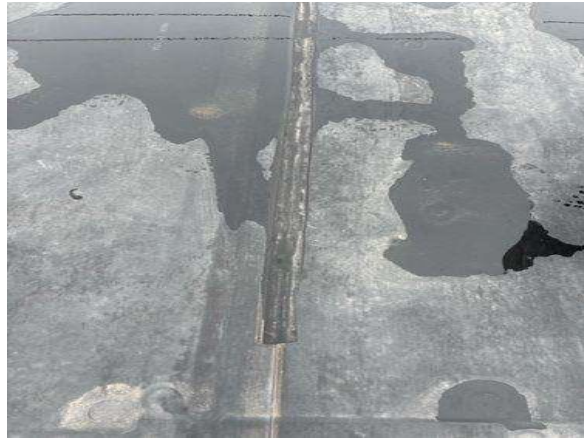
Whoever made these repairs cut 6" cover tape in half to seal a seam. The minimum tape size for an EPDM roof is 6", it should not be any thinner to ensure the seam is sealed correctly.
