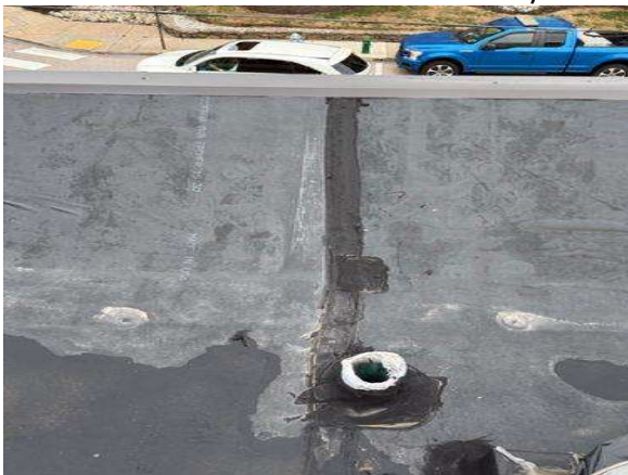
Whoever made these repairs cut 6" cover tape in half to seal a seam. The minimum tape size for an EPDM roof is 6", it should not be any thinner to ensure the seam is sealed correctly.
