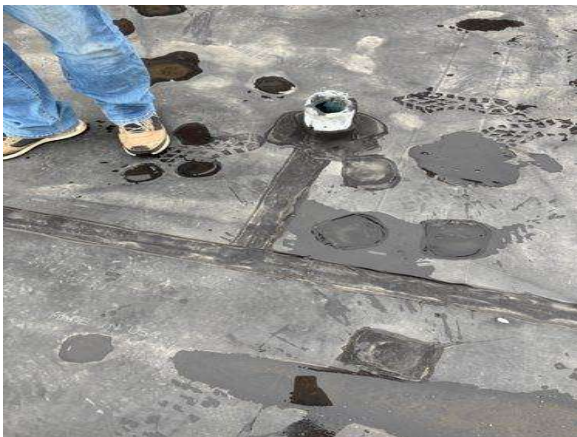
This is not the proper repair to patch an EPDM roof membrane. This should have a proper pipe boot installed.
