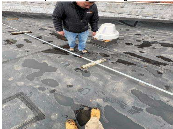
This area has been identified as being soft which indicates moisture under the membrane.
