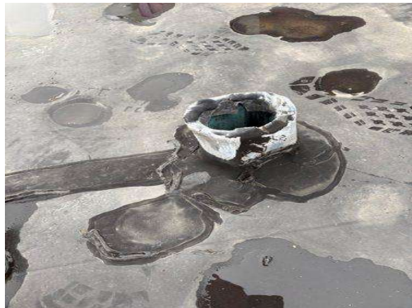
This should have a proper pipe boot installed.
