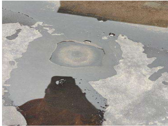
This is not the proper repair to patch an EPDM roof membrane.
