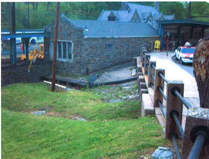
Stormwater conveyance is currently inadequate
